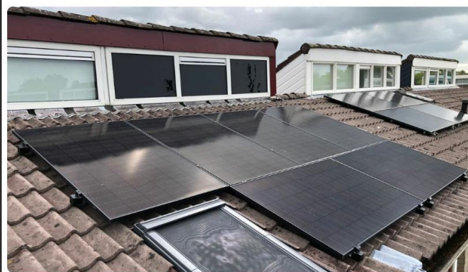
Sinnepanelen op in dak © Energie Service-Noord
